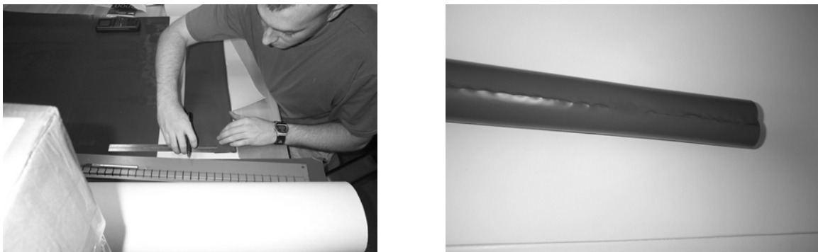
Figure 5.3 Cutting the damping sheet (a) and forming the “damping sausage” with a lap joint
